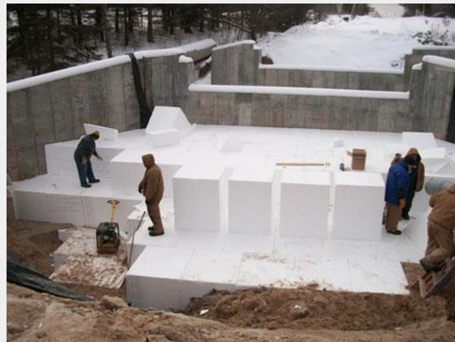
Soil backfill was removed and replaced with geofoam to prevent further damage of the Biscuit Creek Bridge.
