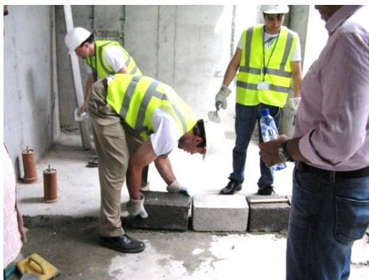
Picture 4: Under the supervision of Mr. Yabroudi, internship participants are learning how to build a masonry blockwall.
