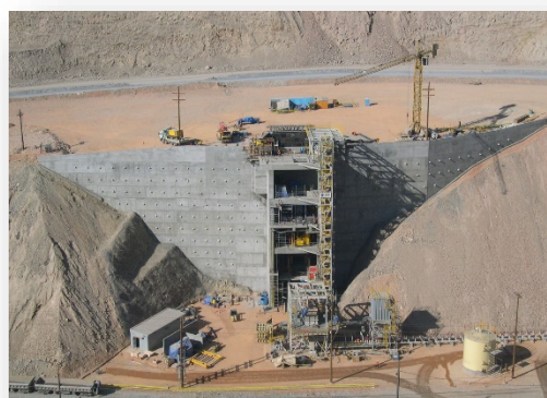
Crusher, Toquepala Mine, Peru
