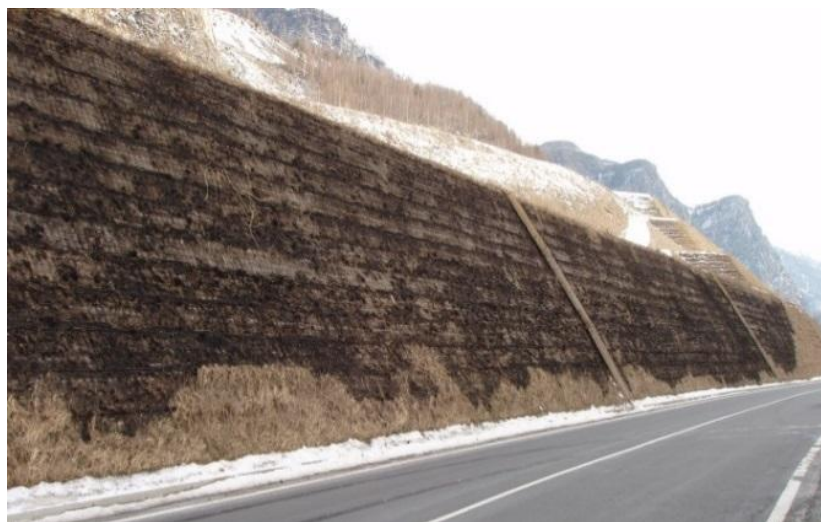
Figure 5 The reinforced structure after the fire event
