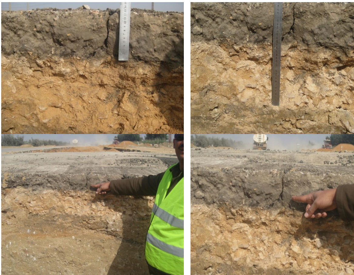
Figure (2): Cracks Extended to Base Layer
