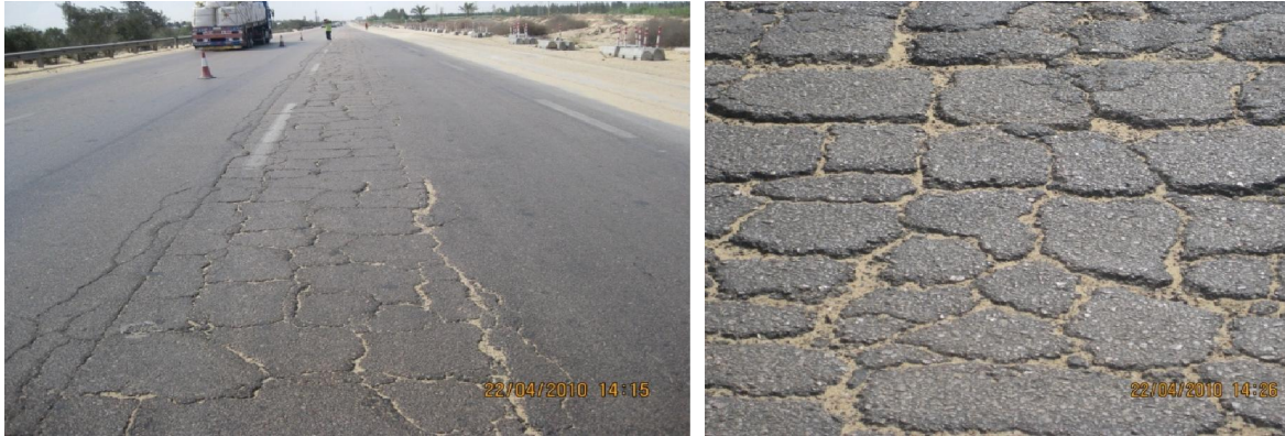
Figure (1): Cairo/Alexandria Freeway Cracks
