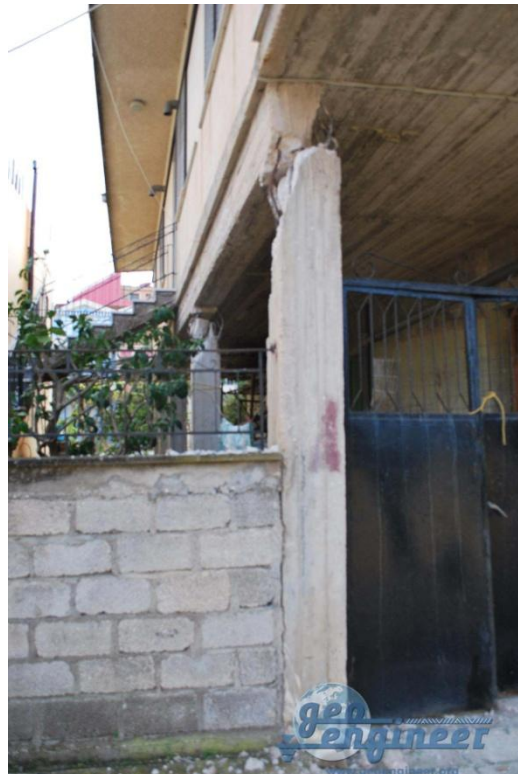
Picture 15: Example of Soft-storey failure
