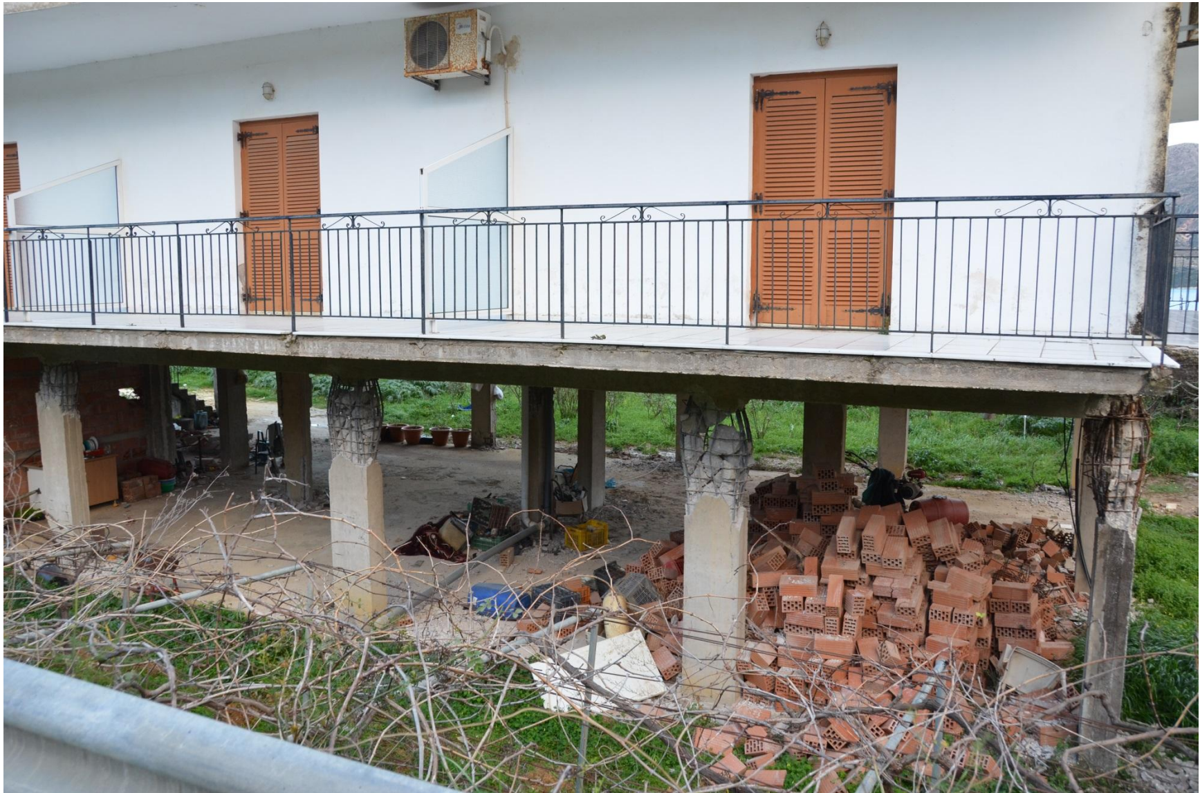
Photo 7. Severe damage to the columns of the 'soft' ground floor of a two-story building at Agios Dimitrios after the second earthquake of Feb. 3. The 'stiff' upper floor suffered no evident damage.
