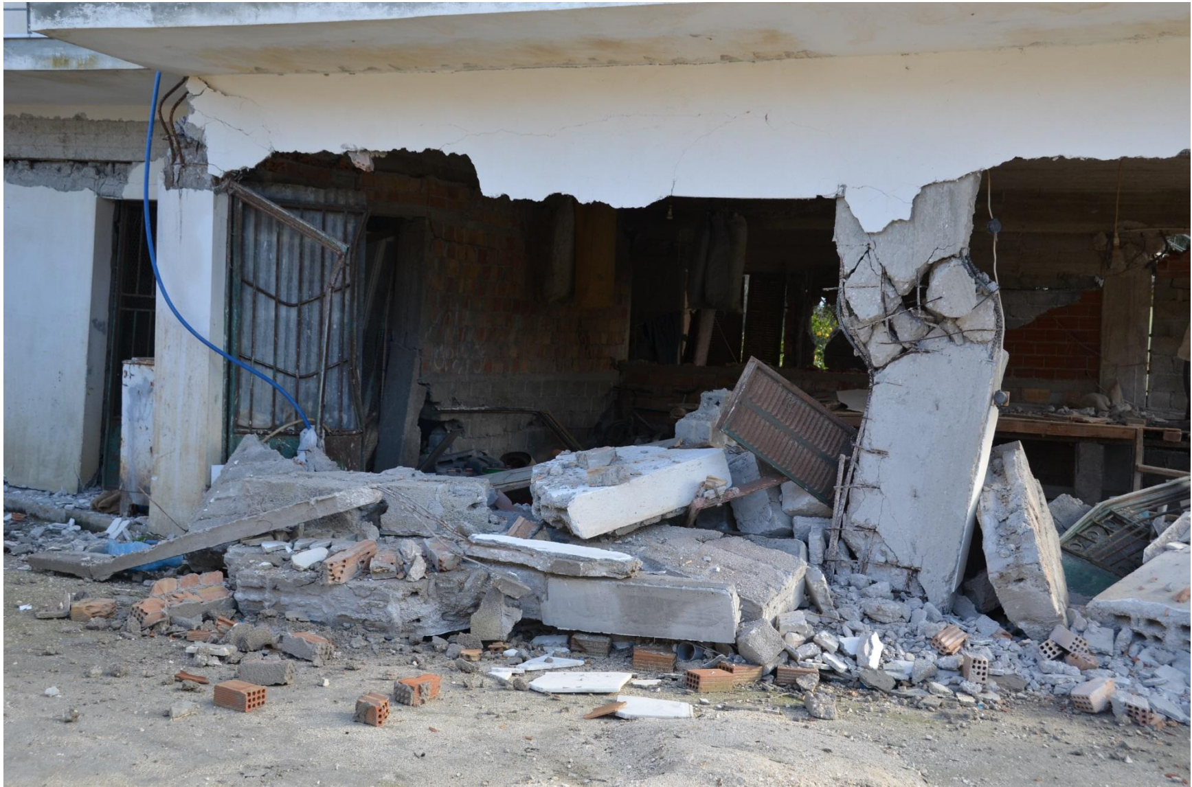
Photo 6. View of the façade of the building of Photo 5 after the second earthquake of Feb. 3: the central column suffered severe damage around the pre-existing shear crack while the infill walls totally collapsed.
