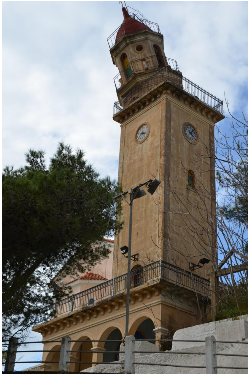
Photo 8. Collapse of the RC columns at the upper part of a bell tower at Kourouklata after the second earthquake of Feb. 3. The lower part of the tower had strong infill brick wall and survived the ground shaking without any damage.
