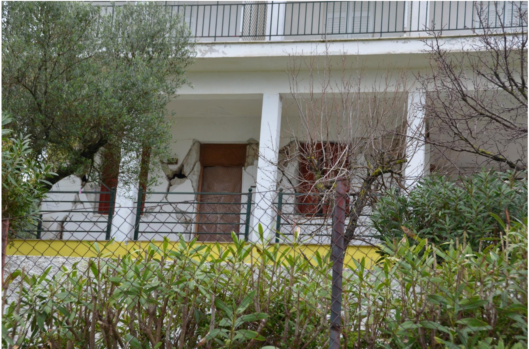
Photo 3. Damaged two-story building at Agios Dimitrios after the first earthquake of Jan. 26. Here shown is extensive damage to brick infill walls. The building suffered limited damage to the RC columns, too ( Photo 4 ).
