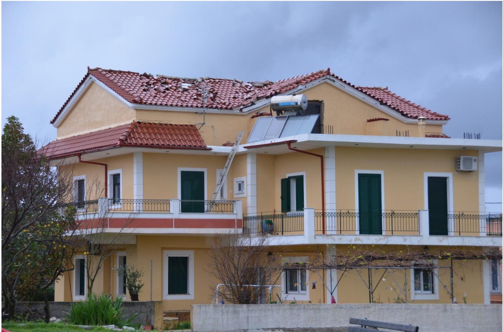
Photo 11. The majority of the houses in the epicentral region suffered no evident damage, or damage to non-structural elements only, caused by the large accelerations developed. Typical non-structural damage was the dislocation of roof tiles.
