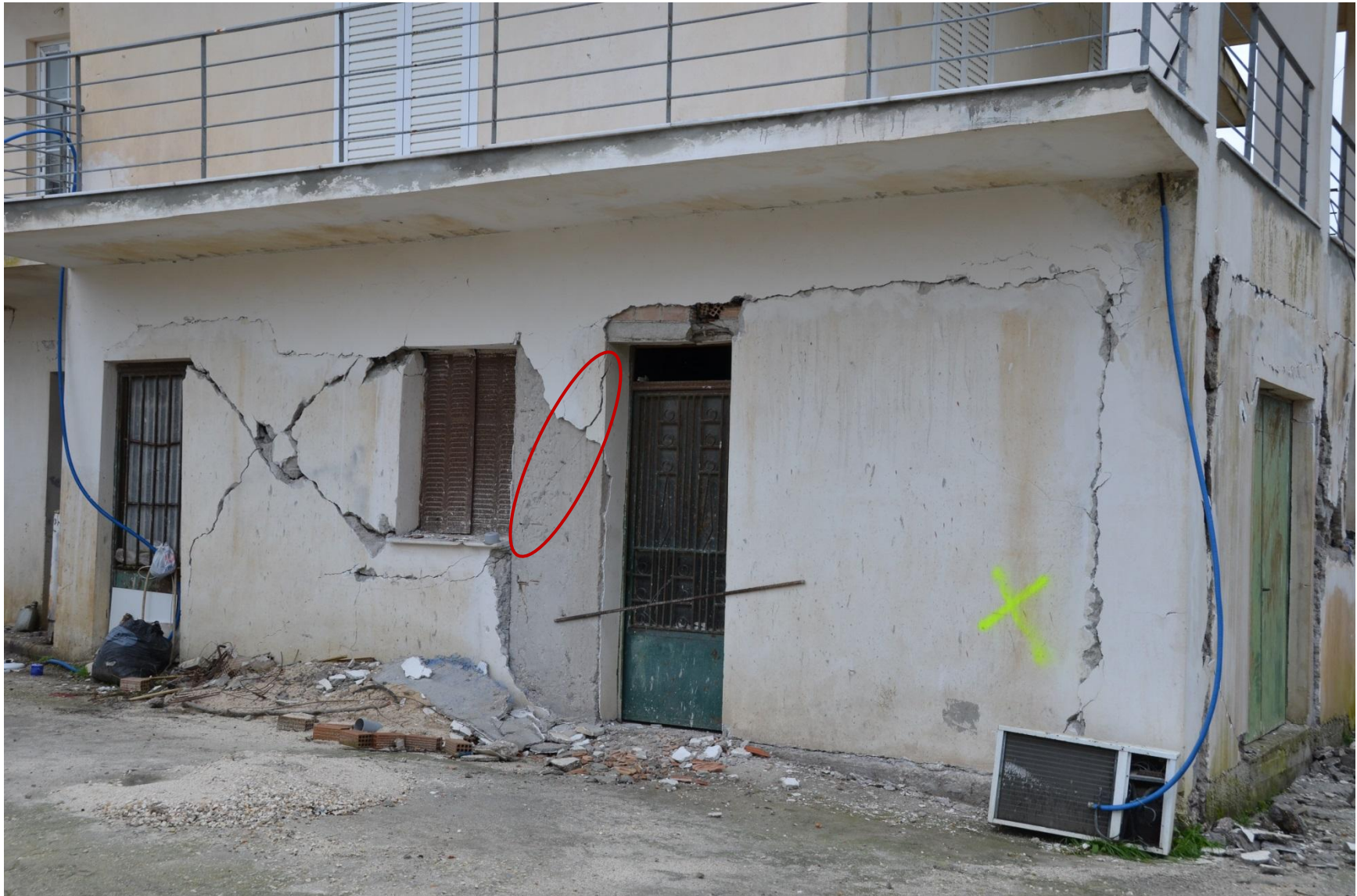
Photo 5. Damaged two-story building at Agios Dimitrios after the first earthquake of Jan. 26: shear failure at the central RC column of the façade (left of the door) and X-shaped shear cracks of infill brick walls.
