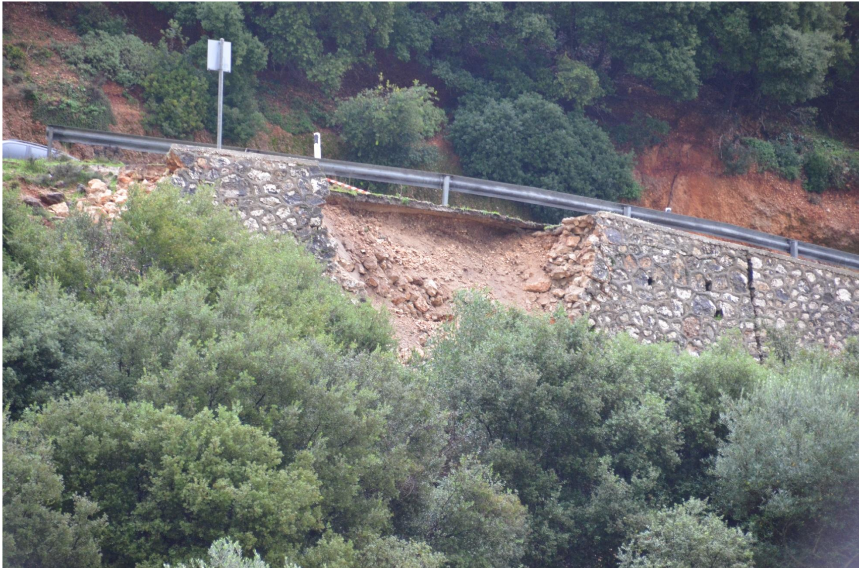
Photo 10. Collapse of an old masonry retaining wall at Kritonou.
