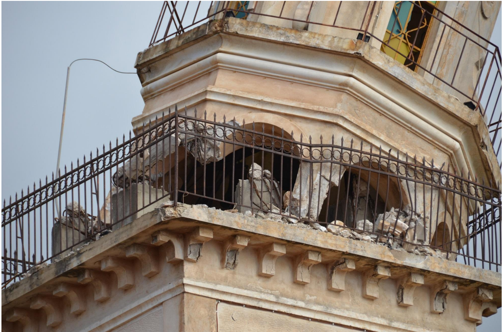
Photo 9. Detail of the collapsed columns of the bell tower of Photo 8.
