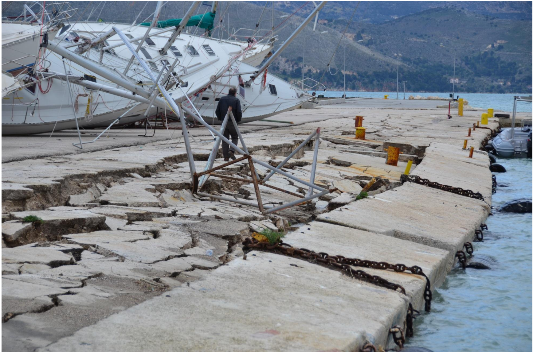
Photo 12. Extensive damage to the quay and inclination of the stones of the waterfront at Lixouri after the second earthquake of Feb. 3. The damage caused to the harbor by the first earthquake of Jan. 26 was very small.
