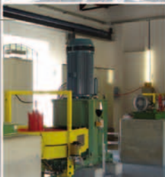
Turbo-generator set of Vessy hydropower plant (Switzerland) Design and project management
